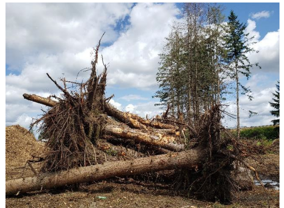
Figure 2: Retention of one hundred trees which will be repurposed as large woody material, providing habitat complexity for aquatic species
