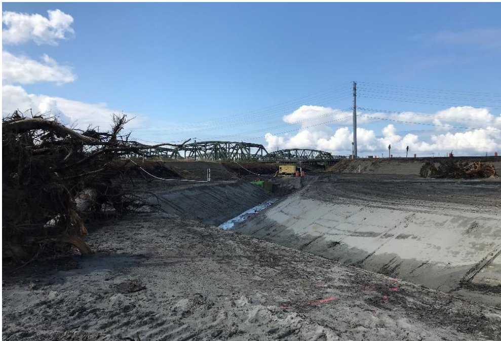
Figure 3: Creation of the new tidal channels which provide: hydrologic connection to Steamboat Slough, salt water conveyance through the mitigation site, accessibility for aquatic and marine species, and habitat for fish including salmonids.
